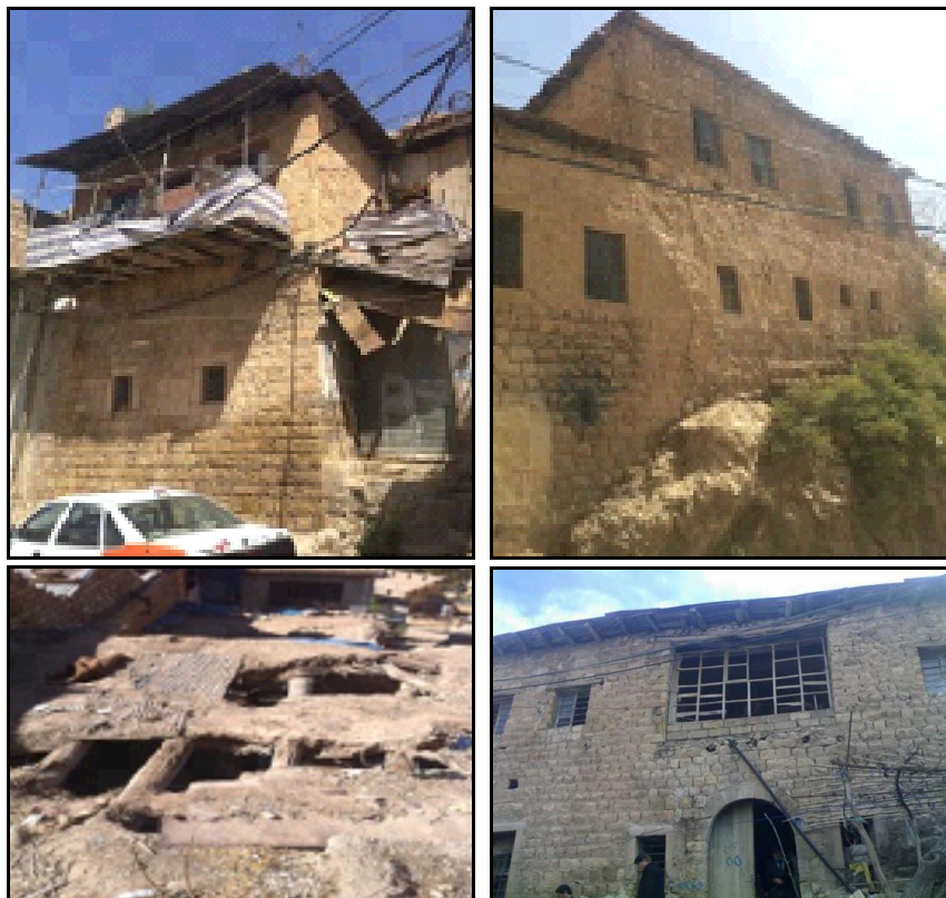
Figure 8-26: Poor condition of the historic houses in Akre city Source: Own photo, Fieldwork, October 2012
