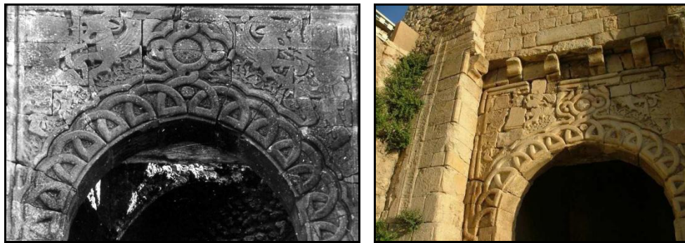
Figure 9-35: Improper restoration of Mosul Gate in Amedy city Source: Amedy Culture Centre, 2007
