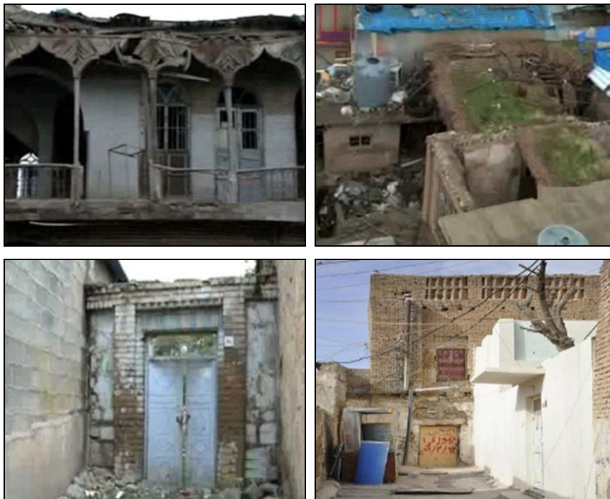
Figure 7-8: Decay in historic buildings in historic centre of Sulaimaniyah Source: NRT Sulaimaniyah Report, 2012
