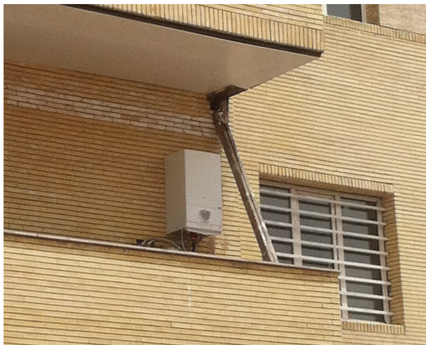
Figure 105: Culture of Cheap Fuel; Water heater is installed in the balcony (Source: Author)
